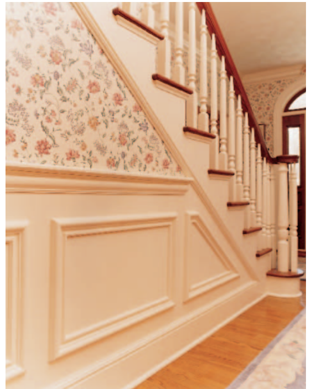
Figure 28-19 Wainscoting Partial Paneling Wainscoting covers the lower portion of a wall. It is sometimes only 32" high and can be made using sheet paneling and molding, or with solid wood.
